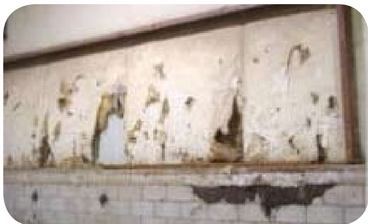
Tremendous Heat Loss w/ Torn Insulation
