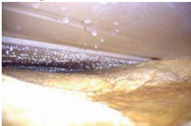
Condensation formed on underside of exterior panel b/c the entire cavity was not filled with fiberglass insulation.
