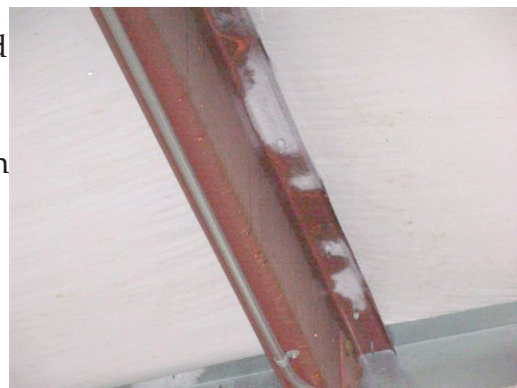
Frost buildup on purlins
