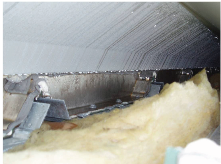
Cold transferred through the metal and formed condensation on the warm air side.
